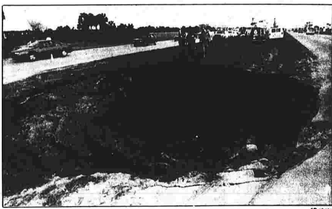
AP photo Police officers and motorists look at a sinkhole about 12 feet deep and 35 feet wide that formed this week in the median of U.S. Highway 192 in Kissimmee, Fla. An engineer with the state said it would take three or four days to stabilize the hole. It will be filled in when it stops growing.
